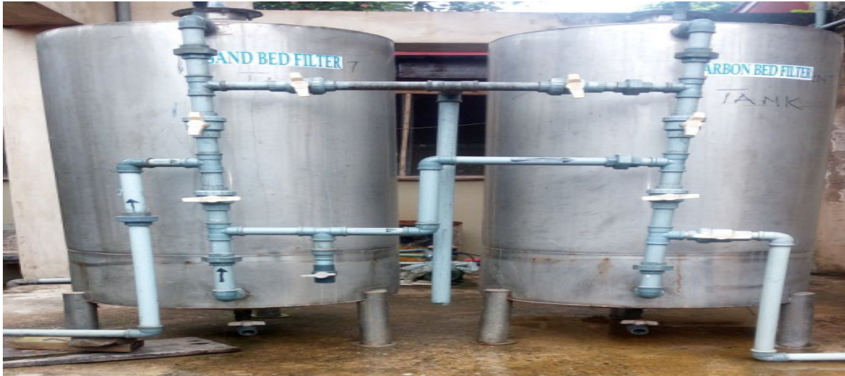
Figure 4: Sand and carbon filters
